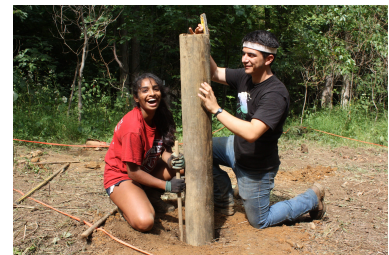
Figure 3.7: We dug and tamped all 3 ft deep post holes for the buildings without power tools.
