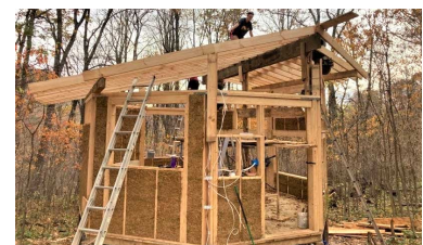
Figure 3.6: Our largest building was octagonally shaped. Building the roof was exceptionally challenging.
